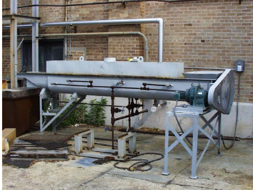
Figure 1-19. Atmospheric Extraction Reactor
